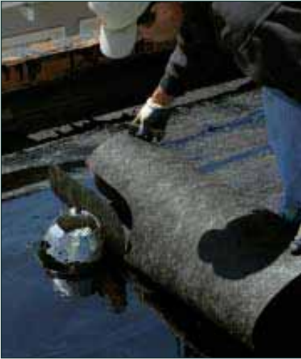
Figure 12. It's possible to flash penetrations after the bulk of the roof is done, but this roofer is laying the roof over the flashings, an approach that creates fewer seams.
