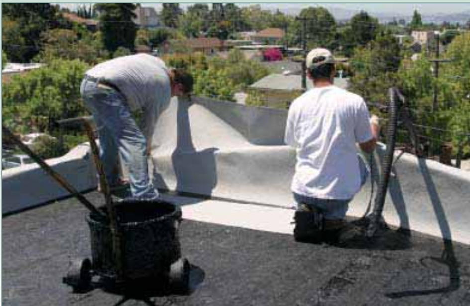
Figure 14. Loose aggregate will not stick to vertical surfaces, so the crew covers parapets with cap-sheet material. The roofers mopped hot asphalt onto the back of the sheet and are flipping it into position.
