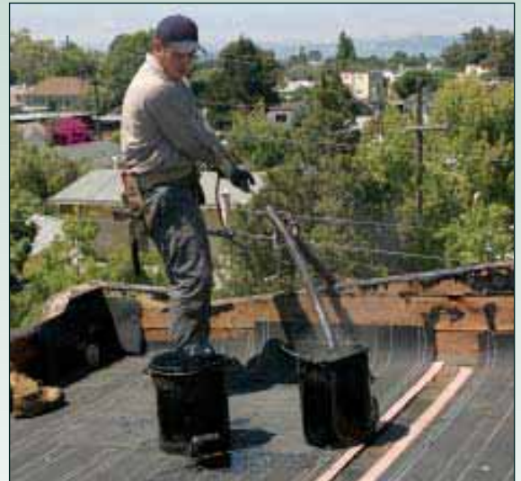
Figure 8. On small jobs, the hot asphalt is carried to the roof in buckets. This job was large enough that it made sense to pump the asphalt up in temporary pipes before transferring it to buckets or wheeled carts.
