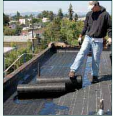
Figure 11. The roofers apply successive layers of felt over hot asphalt. On this roof, full sheets lap \frac{2}{3} onto the sheets below, which means there will be at least three layers of felt plus one layer of base sheet at any given point.
