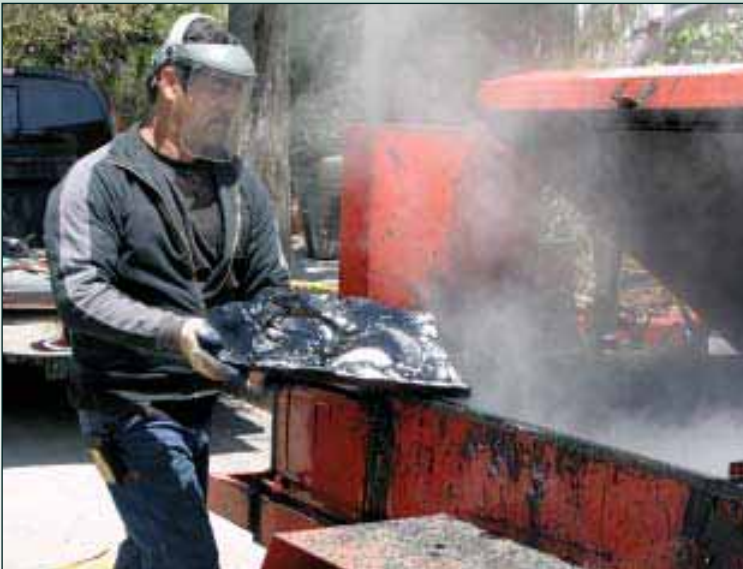
Figure 7. A roofer carefully slips another chunk of asphalt into the kettle. Splashed asphalt can cause serious burns, which is why he is wearing gloves, long sleeves, and face protection.
