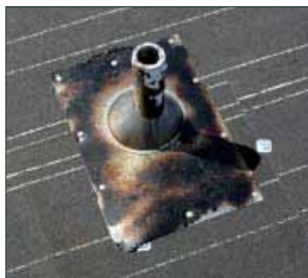
Figure 5. Flashings are primed to make the hot asphalt stick better. Note the caps under the nails that hold the base sheet to the roof.
