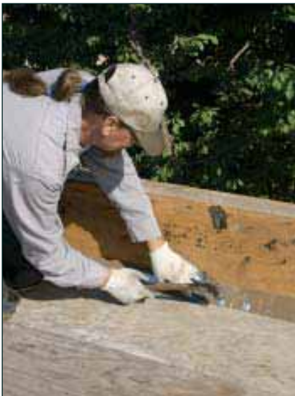
Figure 2. Fiberglass felts will not take tight bends, so the crew installs cant strips at inside corners.
